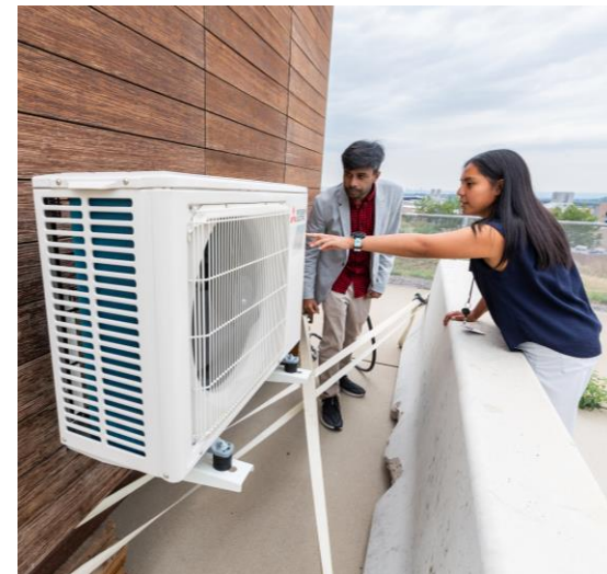
Photo by Werner Slocum / NREL
